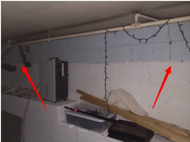
Front of basement, possible hydrostatic pressure
