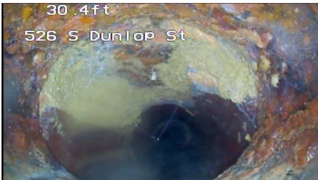
Rust and corrosion on the cast iron portion.
